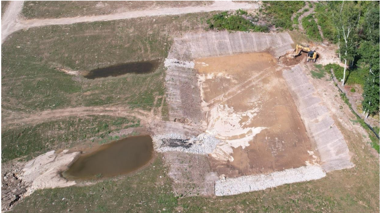
FIGURE 8. Damage to a stormwater basin on the Waterford solar energy site due to heavy precipitation from Tropical Storm Ida, which occurred on September 1-2, 2021.
